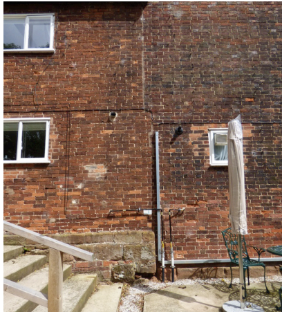
Fig. 2. The chamfered plinth on the original end of the N range, note the straight-line join in the brickwork slightly to the left, above the trunking in the centre of the picture.
