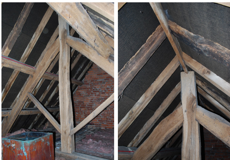
Fig. A3. The early nineteenth century roof structure in unit C (photos James Edgar) (a) Whole truss; (b) Apex of king post (smoke-blackened rafters in foreground)
