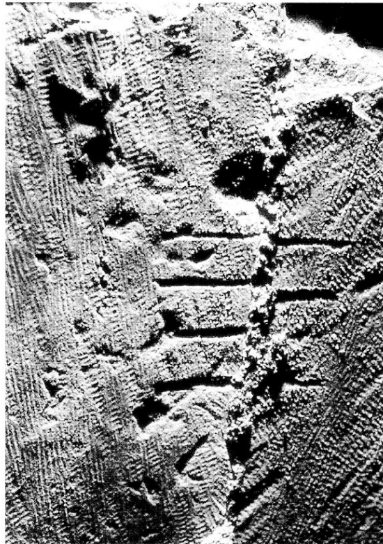
2.4. Joint marks on blocks of stone used in a newel stair of the Lincoln Cathedral Angel Choir, mid-13th century [ Author ].
