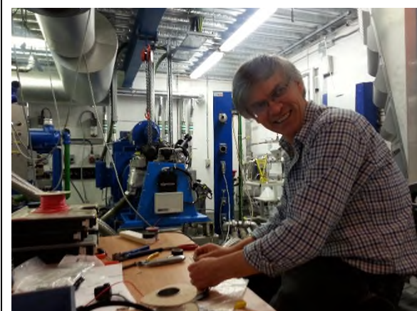
14 Jun 2016: External contractor undertaking bespoke wiring to interface the engine's ECU to the VEF 12V power systems.
