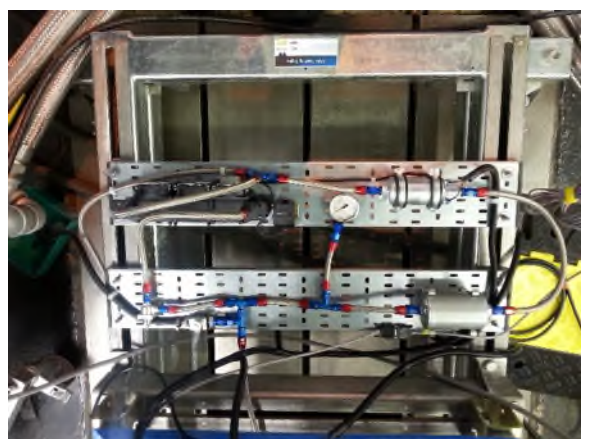
19 Jul 2016: High pressure fuel system showing pump, cooler and fans, filter, drain-off valve, pressure regulator, pressure guage and engine run time hours meter.
