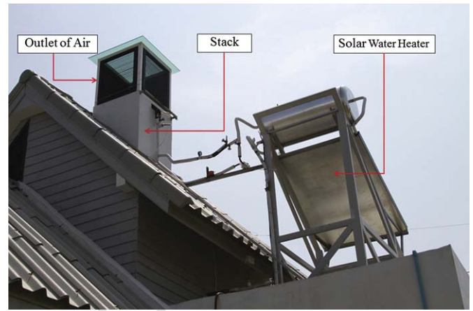
Fig. 2. Light pipe and solar heated ventilation stack.
