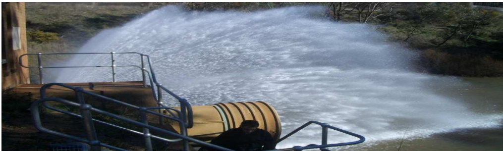
Figure 1.3: Top: Picture of a fixed-cone valve. Bottom: Picture of water release from Lake Nillahcootie.
