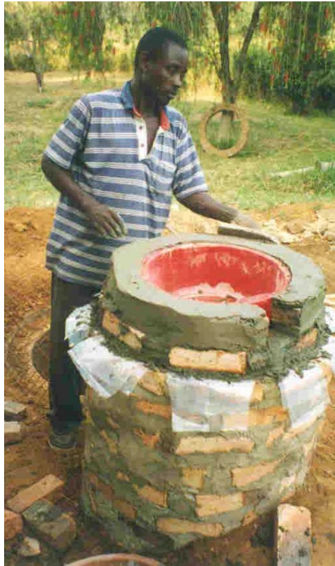
Figure 6 Applying render to the top course with the basin in situ, notice the gap left for the handpump
