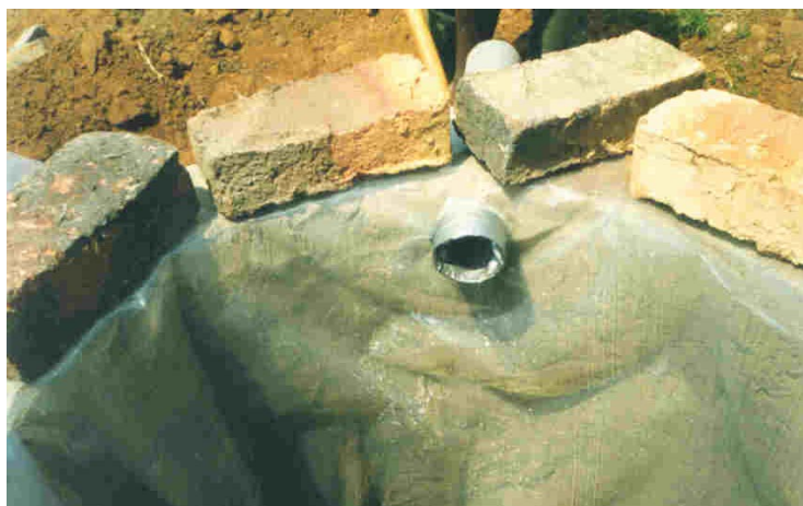
Figure 5 The plastic is folded over on top of the parapet prior to the next course of bricks
