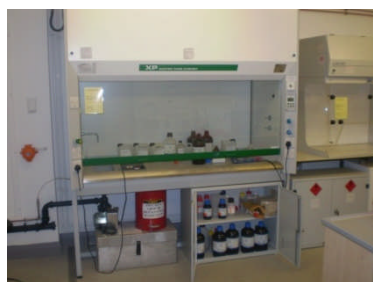
Fume hood and solvents cupboard
