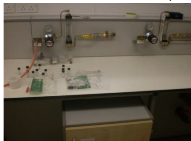
Compressed air and nitrogen supply
