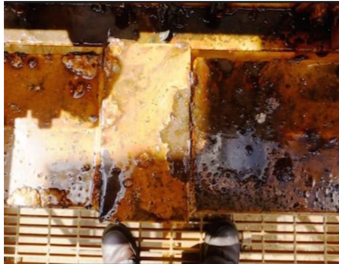
Saline-Induced Corrosion and Tracking
