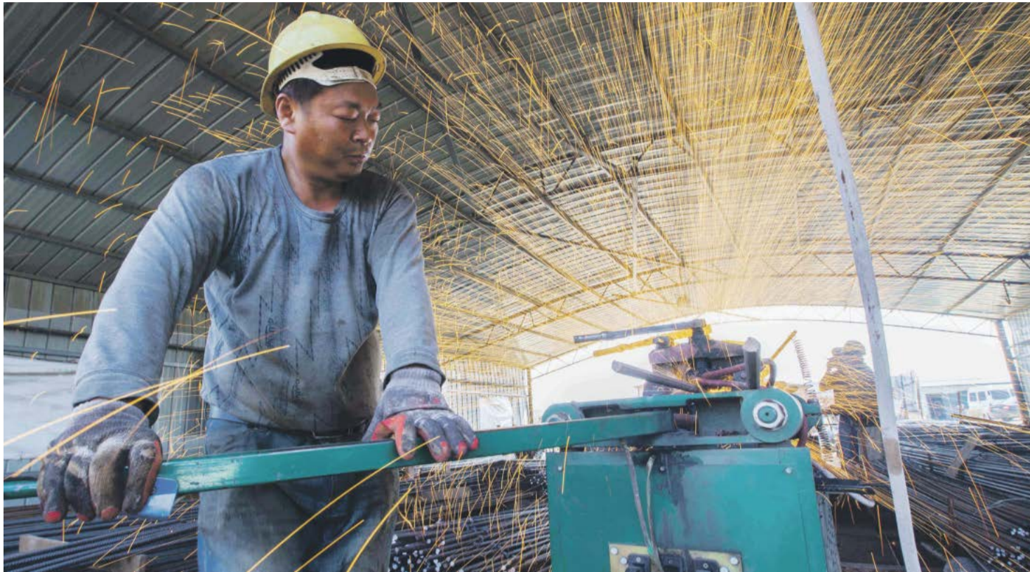
A labourer cuts steel bars at a railway bridge construction site in Lianyungang, Jiangsu province, China. As data points to a cooling in the world's second-largest economy China is planning to clean up and integrate some state firms.
