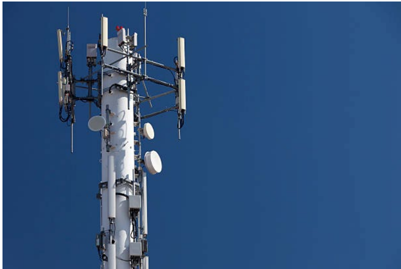
Base station tower
