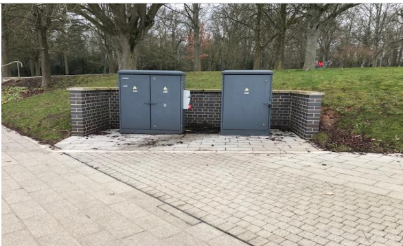
High voltage maintenance boxes.
