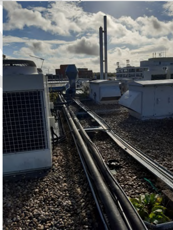
Main roof: trip hazards – uncovered cable trays
