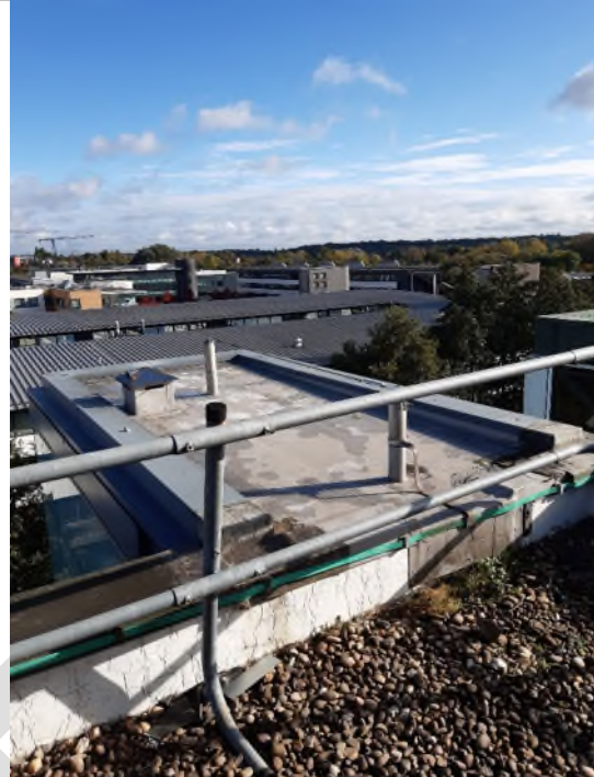
Roof section with man safe system and no edge protection
