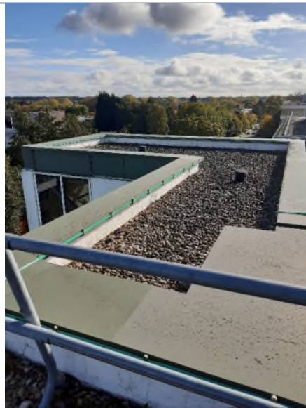
Roof section with no edge protection
