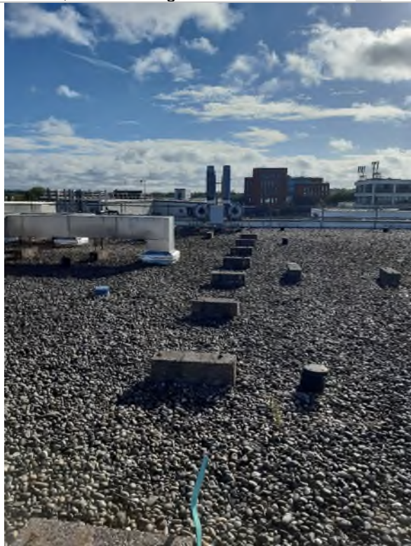
Main roof with trip hazards
