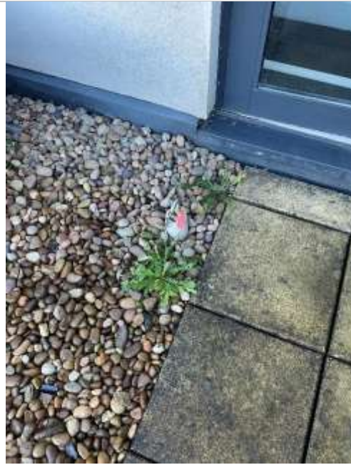
Redundant latch line posts at ground level
