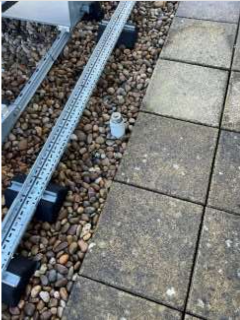
Redundant latch line posts at ground level
