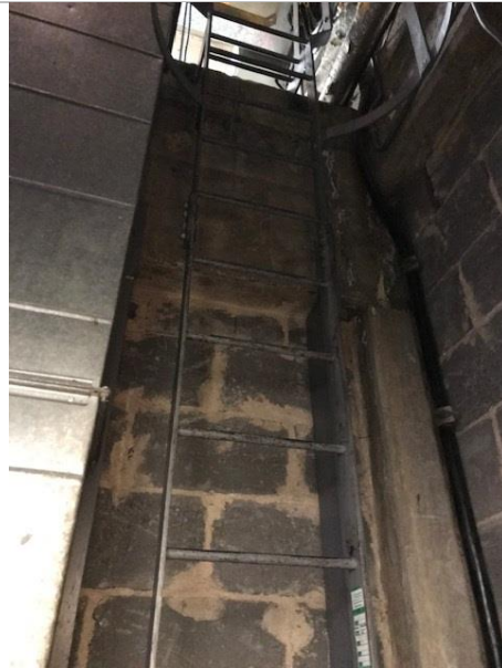
Galvanised steel fixed ladder
