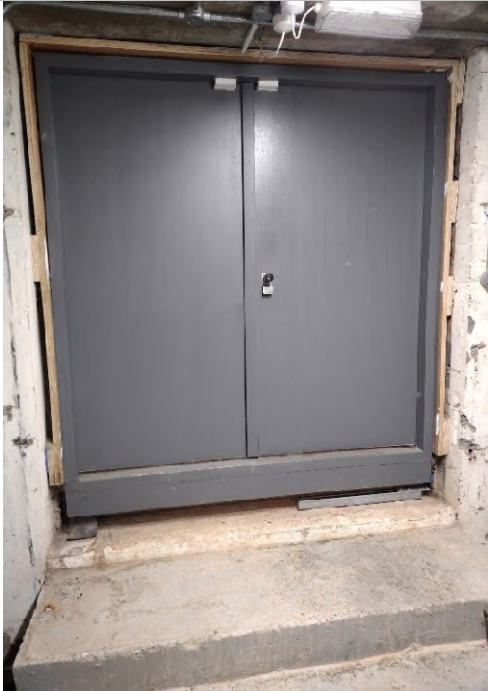
Roof access door with Salto barrel
