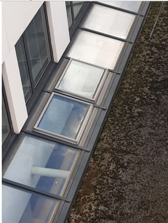
Roof lights and smoke vents on atrium roof
