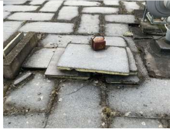
Loose slabs causing trip hazard along with resulting holes at floor level
