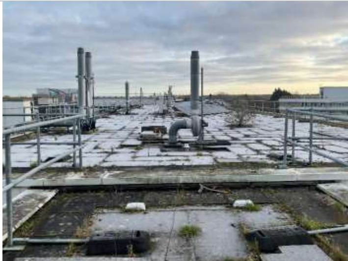
Roof overview, trip hazard edge protection weights
