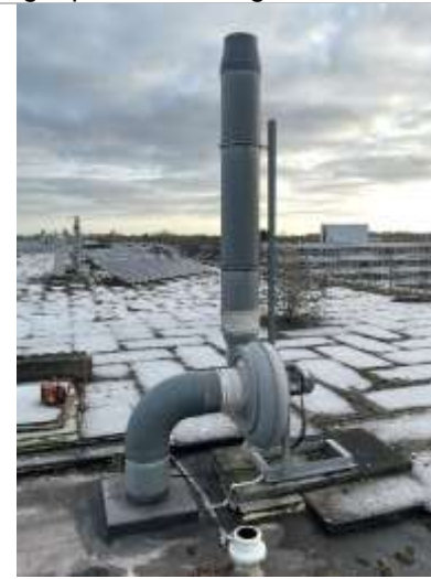
Typical Chemistry/Engineering flue
