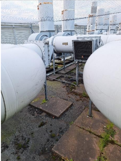
Example of narrow space between ducting
