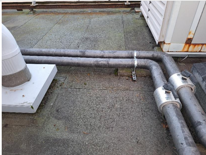
Pipework at floor level
