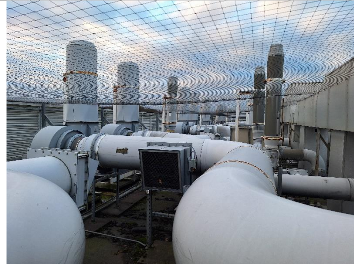
General plant and ventilation
