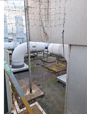
Head height duct work
