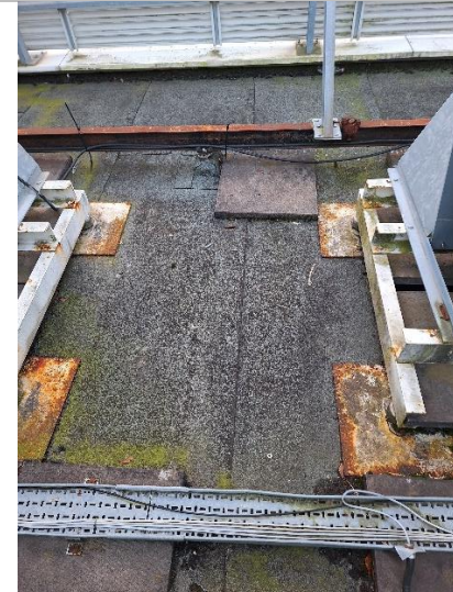
Example of raised slabs and cable trays
