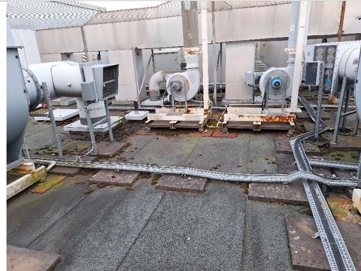
Typical plant and cable trays
