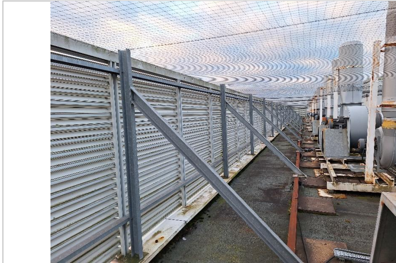
Example of edge protection
