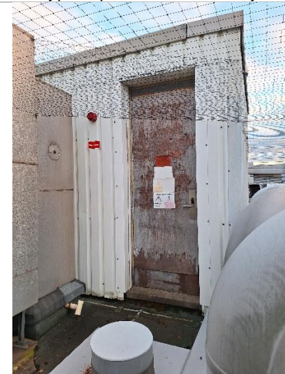
Lift motor room access door (Salto)
