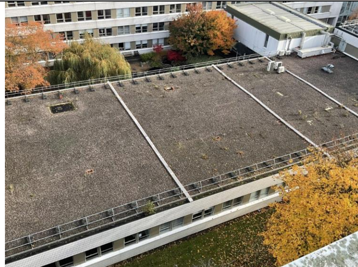
Lower block roof (RAAC)
