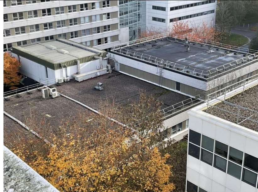
Lower block roof (RAAC)
