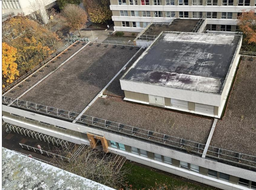
Lower block roof (RAAC)
