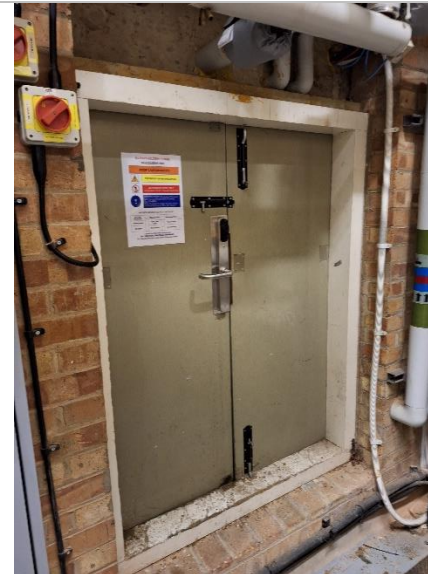
Roof access door in plantroom (SALTO)
