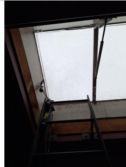
SALTO padlock on roof hatch
