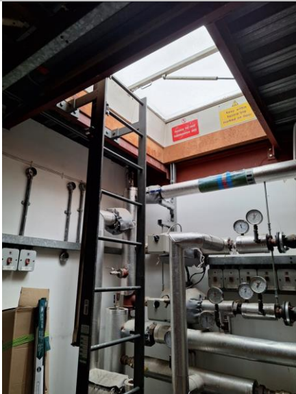
Roof access ladder
