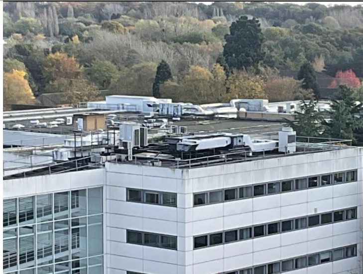
Humanities Extension roof plant
