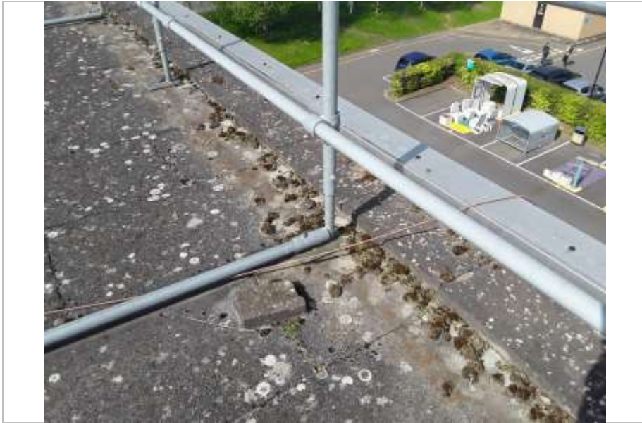
Edge protection supports not anchored
