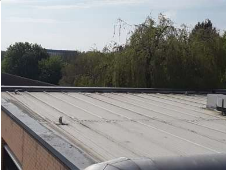
Area of roof without edge protection
