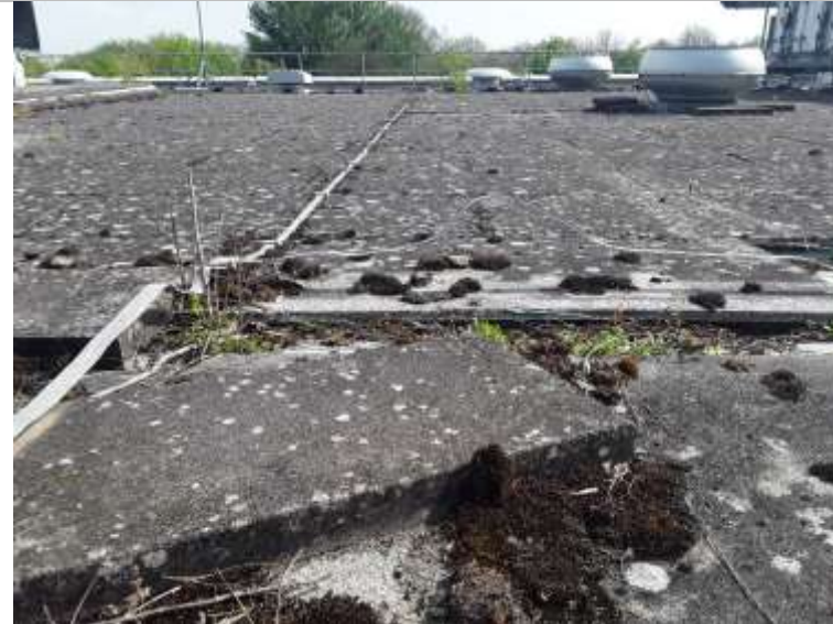
Typical loose slab along with raised lightning conductor cable
