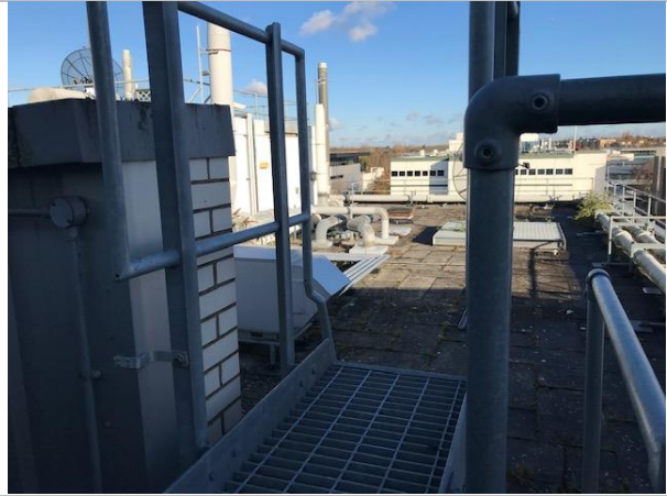
From the live in roof you can also access the Physics roof from the live in roof.
