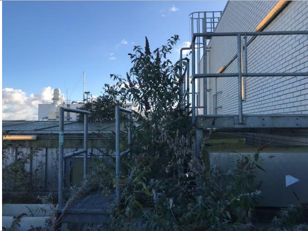
Overgrown vegetation on the live in roof.
