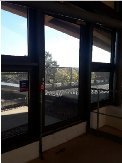
Roof access door
