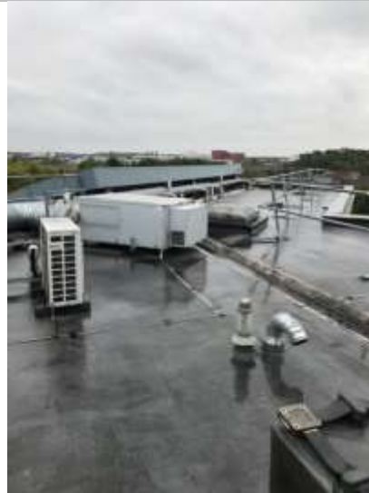
Plant Equipment on roof
