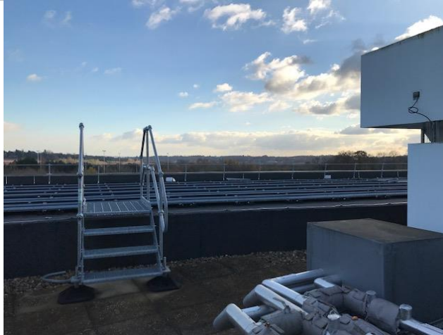
Steps leading to roof with PV Panels
