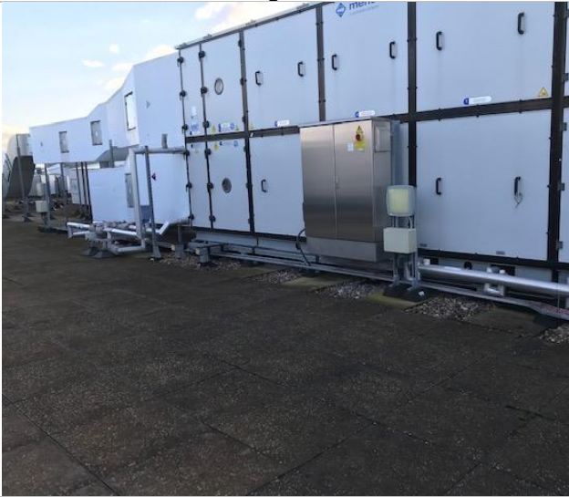
External roof machinery and plant
