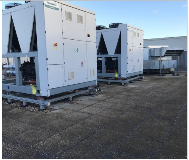
External roof machinery and plant
