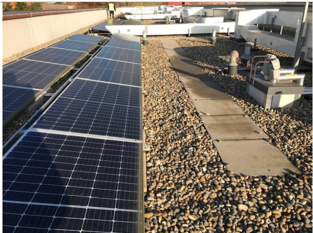
Cryfield 8 External roof PV Panels.
