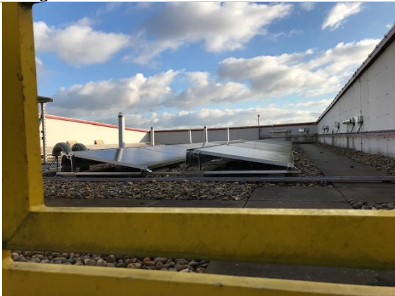
Cryfield 6 PV Panels on higher level roof
