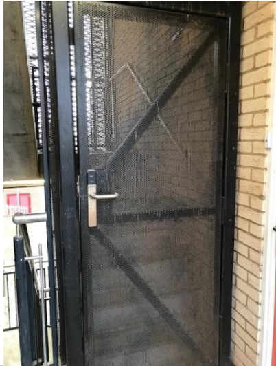
Cryfield 5 Salto access gate on the 1 st Floor and the 3 rd Floor
