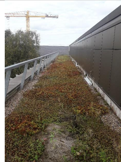
Vegetation growing, causing potential trip hazard and loose ballast
