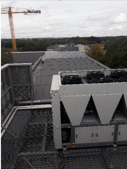
Example of typical plant
